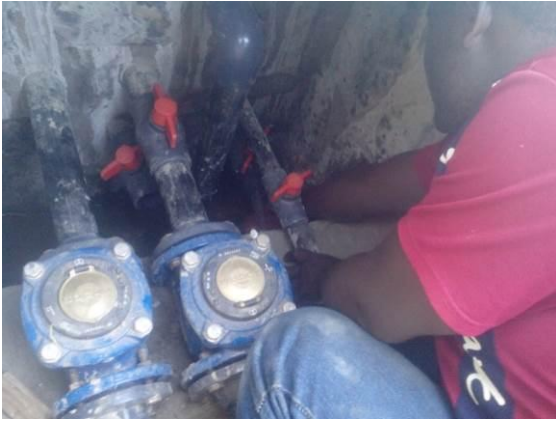
Main water meters
